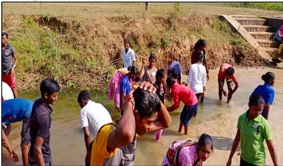
Fig.: NSS volunteers constructing check dam of sand bags on sewer (Nala) near Pujaripara of Kerawahi village.
