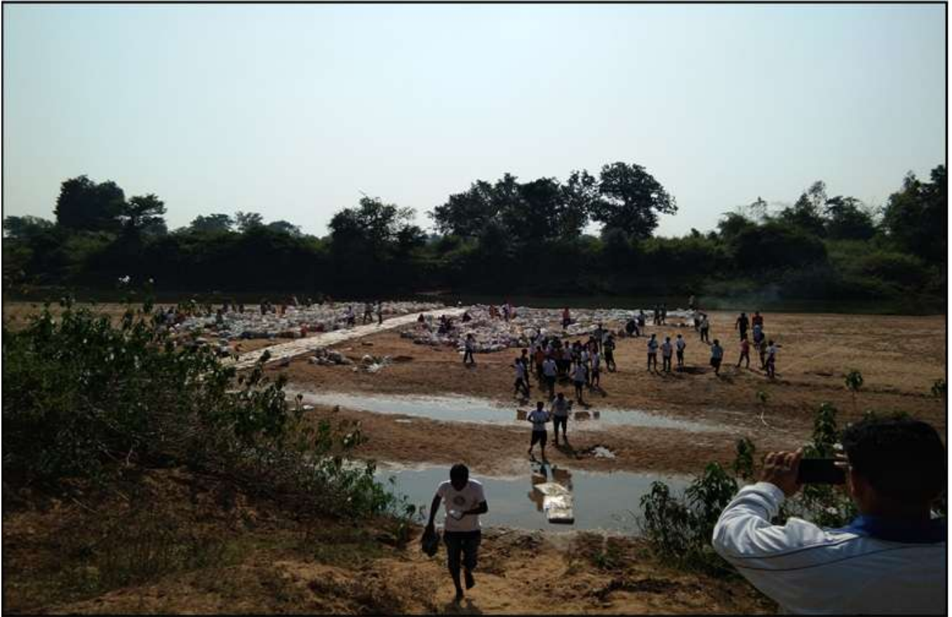
Fig.: NSS volunteers constructing check dam of sand bags on Narangi River near funeral place of Kondagaon.
