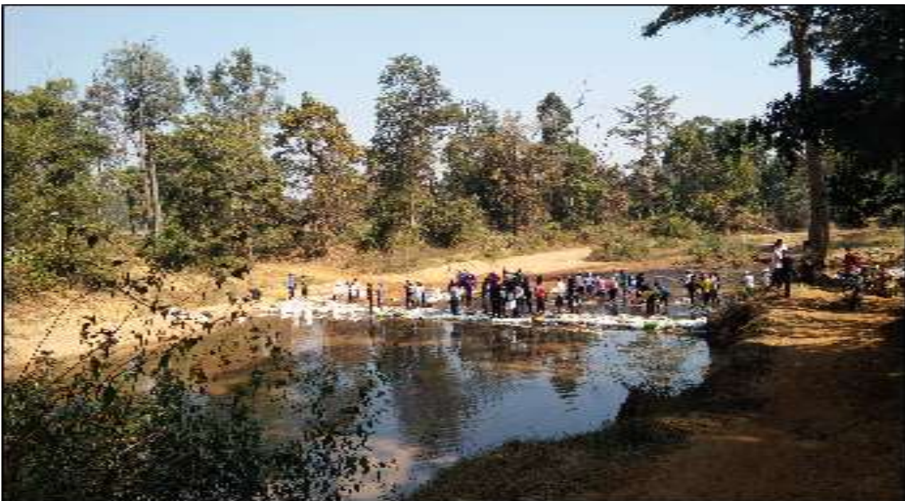
Fig.: NSS volunteers constructing check dam of sand bags on Latura River near Buddha Chaitya place.
