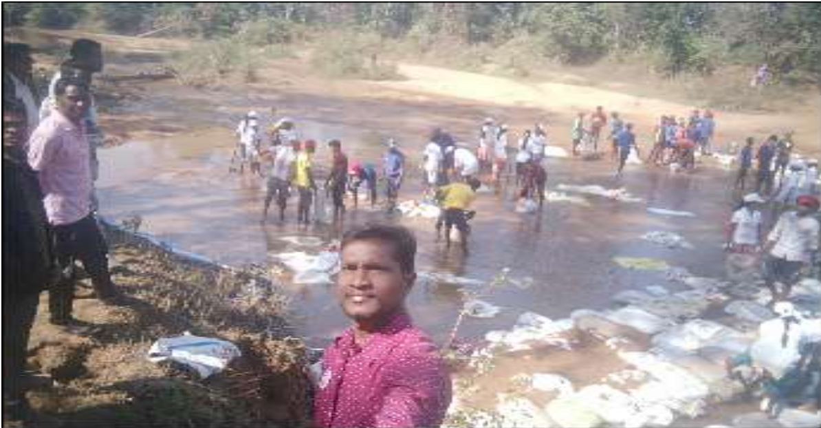
Fig.: NSS volunteers constructing check dam of sand bags on Latura River near Mishri village.
