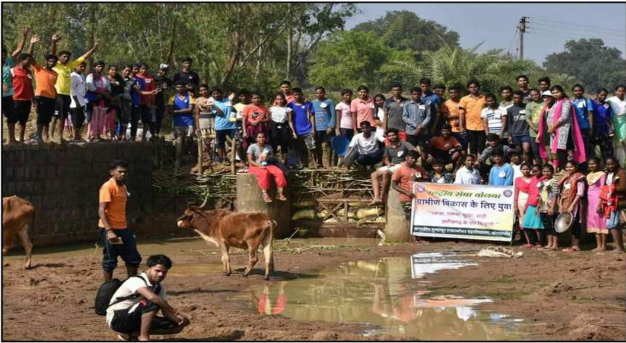
Fig.: NSS volunteers after construction of check dam of sand bags on sewer (Nala) near Pujaripara of Kerawahi village.
