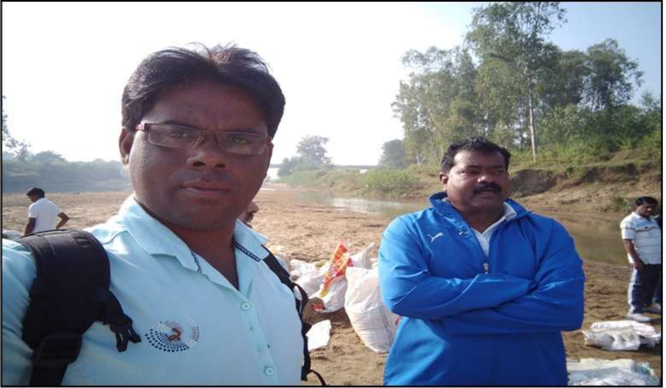
Fig.: NSS Program Officer Mr. Shashibhusan Kannouje and District Magistrate (Collector) Mr. Nilkanth Tekam during construction of check dam of on Narangi River near funeral place of Kondagaon.
